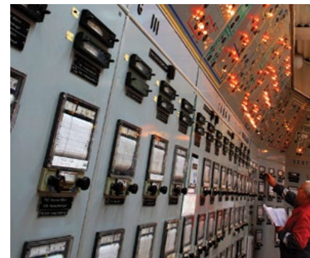
Sterownia w plockiej petrochemii /Petrochemical plant in Plock, control room
